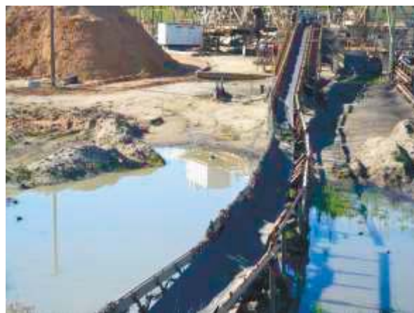
Fig. 5. Damaged conveyor belt
