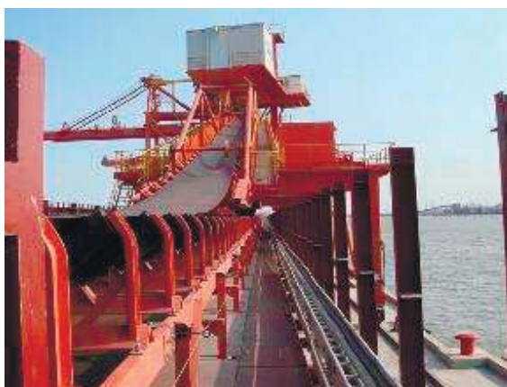
Fig. 1. Belt conveyors in Jiangsu Taicang Environmental Protection Power Plant
